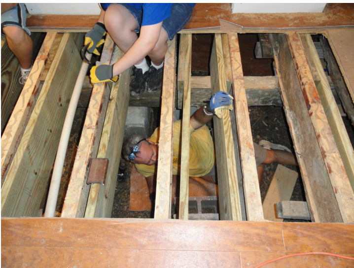
Installing the new floor joists in the crawl space under the floor
